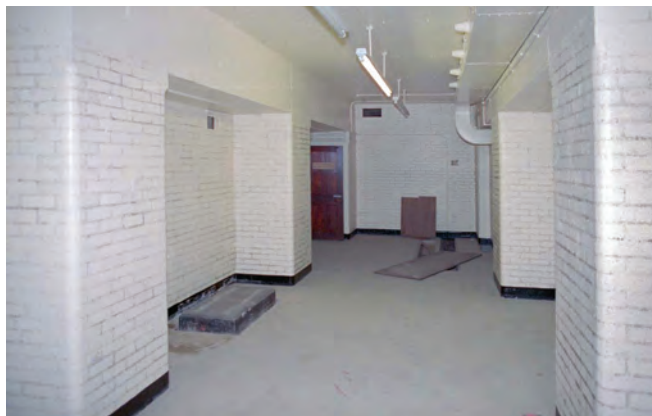
The automatic exchange apparatus room looking west mid-1980s. The door at the back of the room is into the generator room. Note brick pillars which surround the original cast iron columns in the N warehouse basement. Photo from Sub Brit Collection
